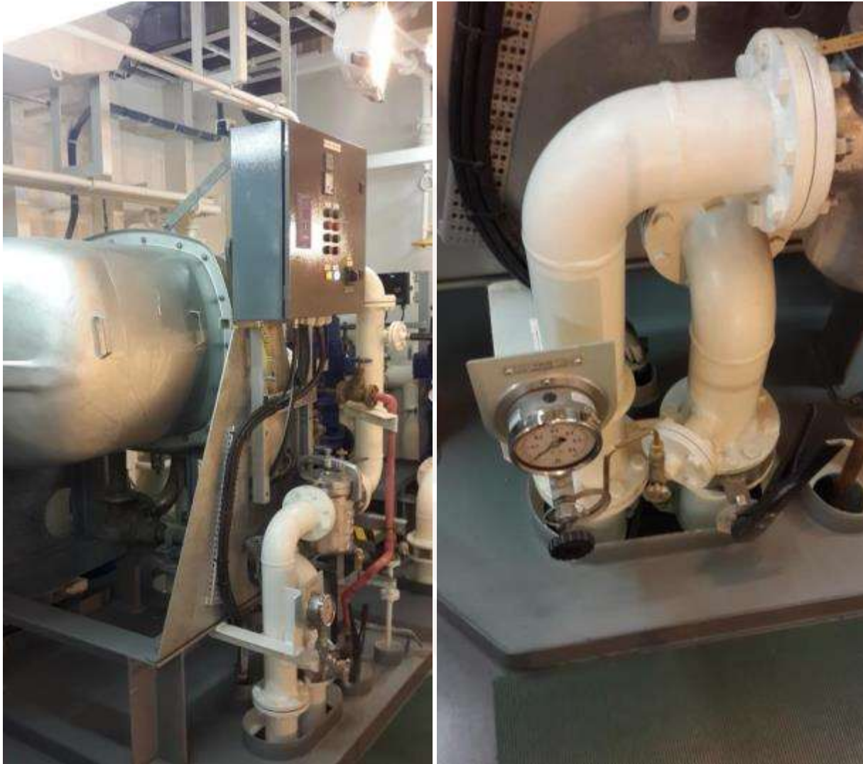
Figure 2. The Fresh Water Generator with its inlet and outlet pipes (inlet is the right pipe on the right photo)
